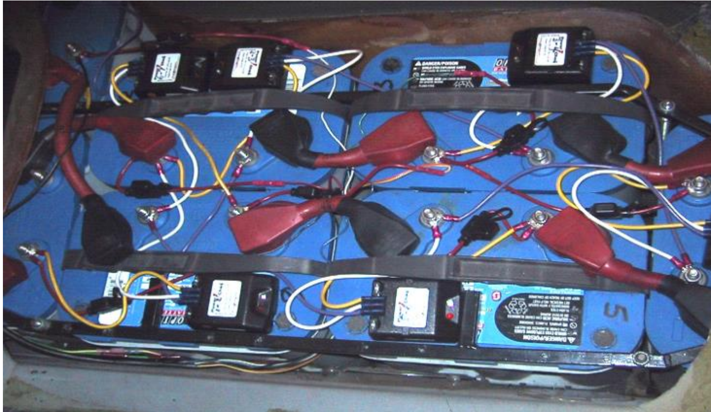
Optima Blue Top AGM Sealed Lead Acid Batteries with PCHC-12V-2A Power Cheqs Installed in a Corbin Sparrow
