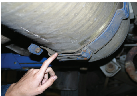
Check for Signs of Cylinder Movement
