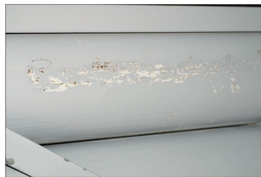
Corrosion and Peeling Paint on Type 1 Cylinder
