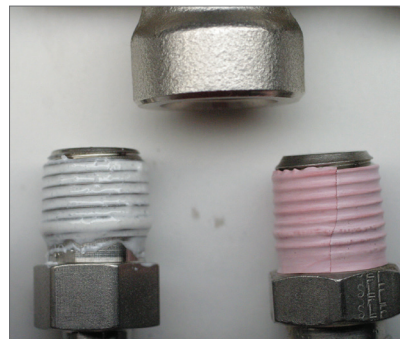
High Pressure Fittings must be Carefully Sealed and Assembled
