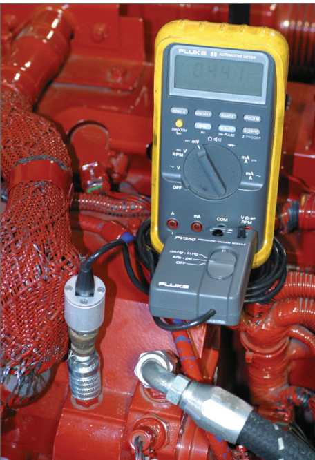
Electronic Transducer on Meter
